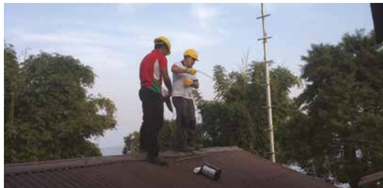
Cpl Khagendra and LCpl Prakash maintaining HF antenna, AWC Bhojpur
