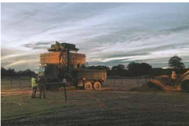
Filling the top layer of the Expeditionary Elevated Sangar using a Self-Loading Dump Truck
