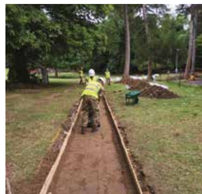
I Troop - Constructing a foot path and a gap for the bridge training at Invicta Park Barracks Training Area
