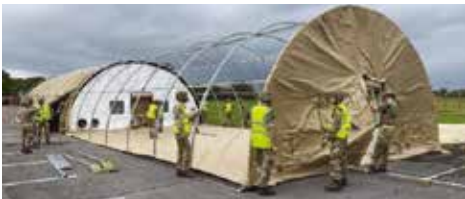
TDA construction for centralised feeding during Ex LOYAL LEDA 20 at South Cerney
