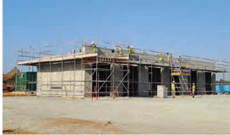
70 Gurkha Field Squadron building a Boat store in Cyprus as part of Adventurous Training facilities refurbishment
