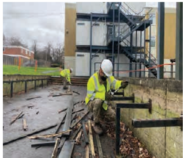
Refurbishment of seating area next to Dundas Block led by Cpl Ganga
