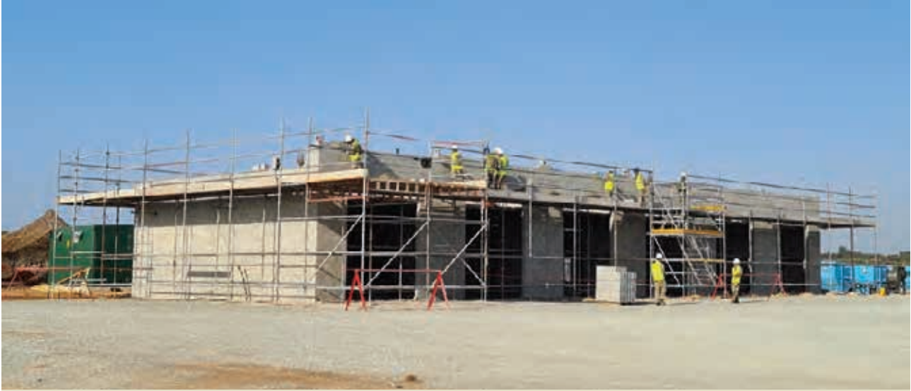
Construction of Boat Store led by SSgt Joseph (Tp SSgt L Tp) on Ex PINESTICK 21
