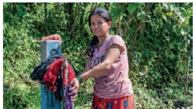
Installing tap stands for every household reduces the burden on women and children who used to travel for hours to collect water
