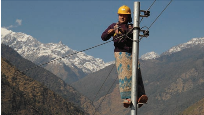
Women are just as capable as men. Installing electric lines at Tumsika, Gorkha
